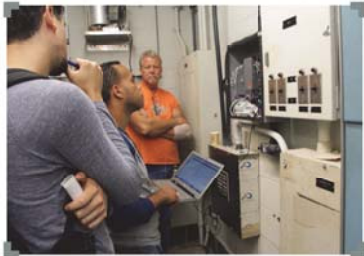
Felix Rodriguez, BPL Equipment Specialist, installs data loggers at a Department of Environmental Protection facility as part of a DCAS-supported research project
